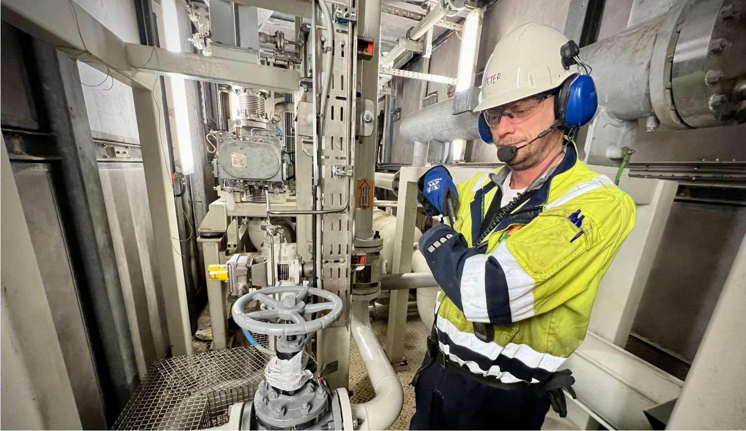
Peter Kongstad Schmidt stands beside the pipe and valve, central components in the VOC to flare project.
