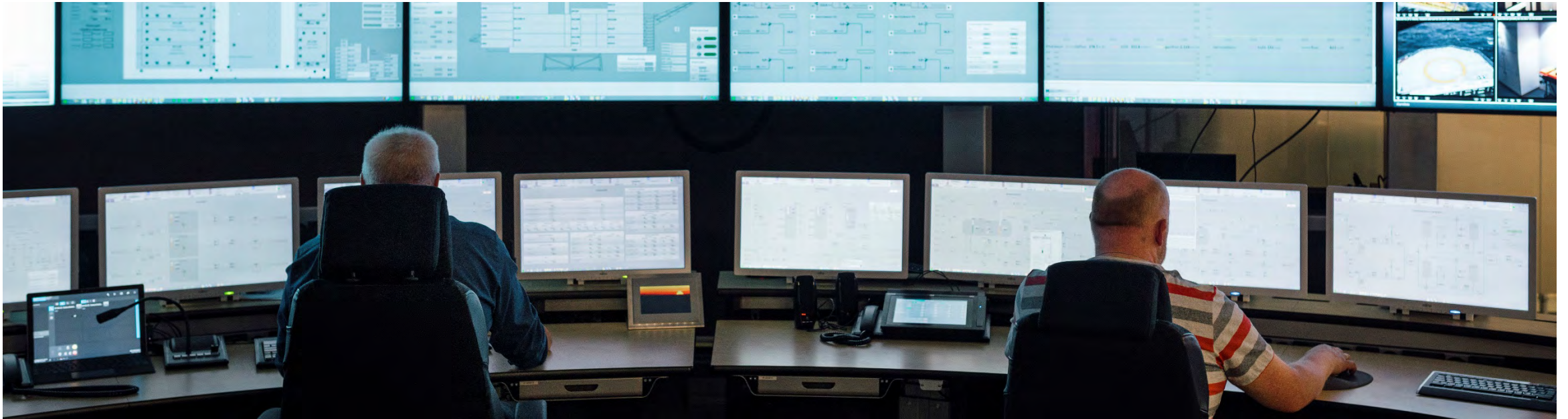
The offshore control room moved onshore as the first in Norway
